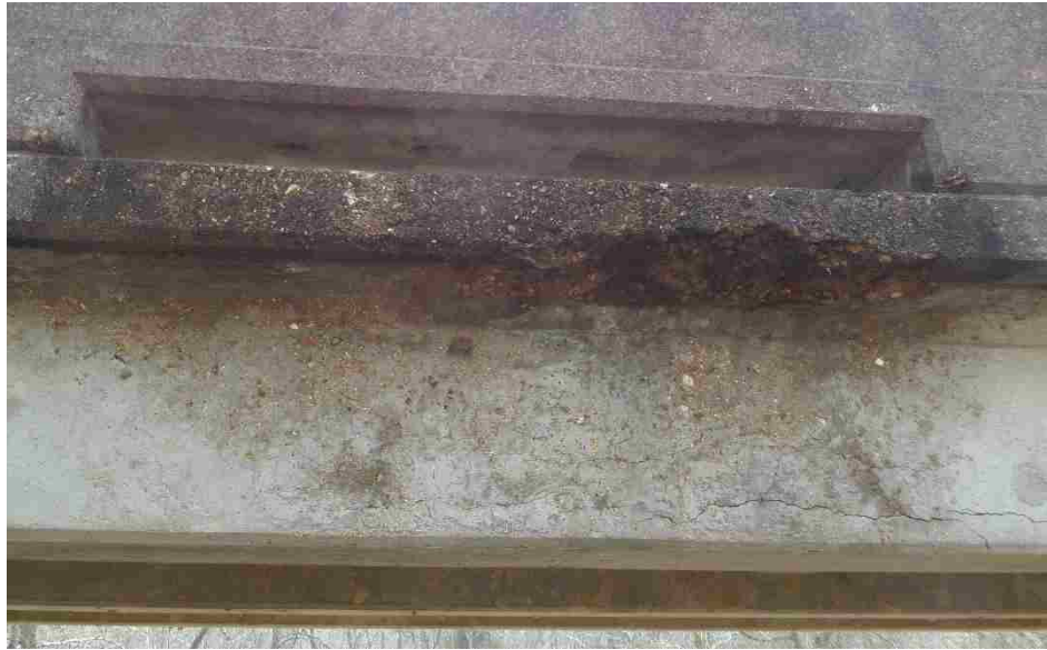
Figure 4.1. Spalling on Girder
